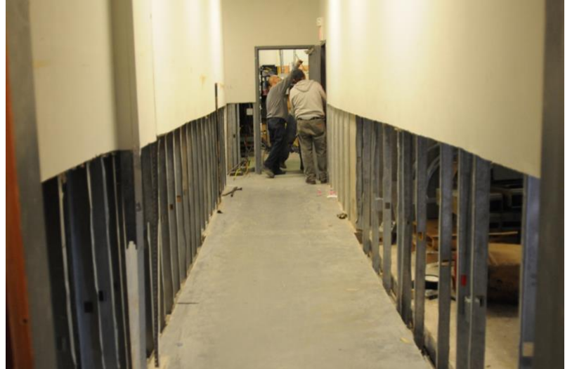
Figure 7: Workmen Cut Out Walls at Flood Damaged Commercial Building (FEMA Photo by George Armstrong)
