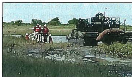
Crews inspect the thin-layer placement site on Jekyll Island in the marsh off Jekyll Creek.
