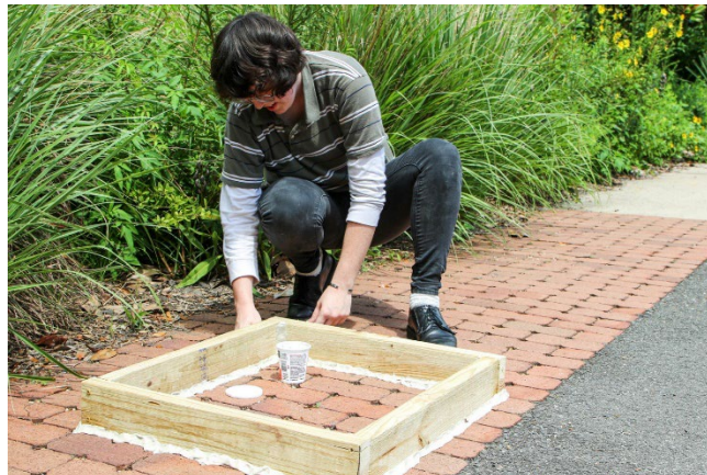
Figure 2. Intern, Jade Bailey, applying 1-inch bead of plumber's putty to SIT infiltrator
