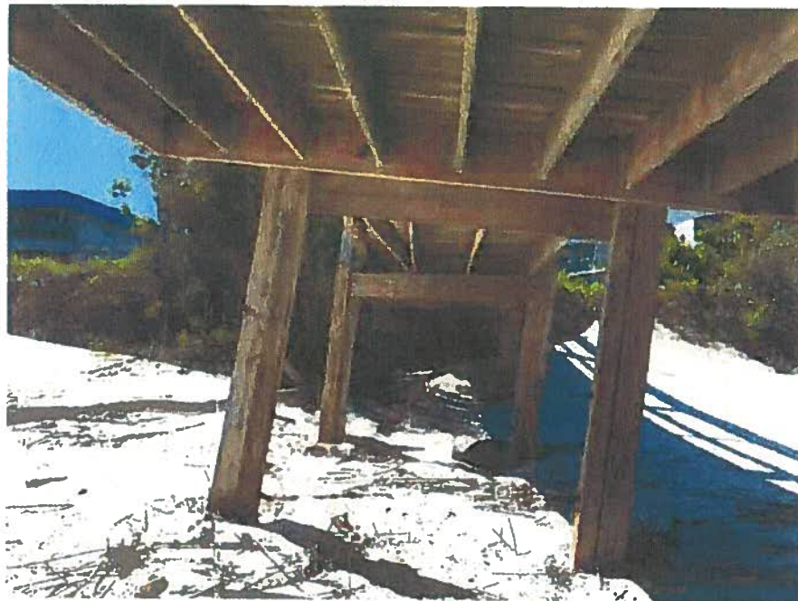
Figure 8 - Underneath view of structural pilings. Beach pilings are 5.5" x 5.5" posts with thru-bolts to 5.5" x 3.5" posts, spaced approximately every 9 feet. Dune pilings are 5.5" x 3.5" posts with 2" x 4" cross-bracing, spaced approximately 10 feet apart.
