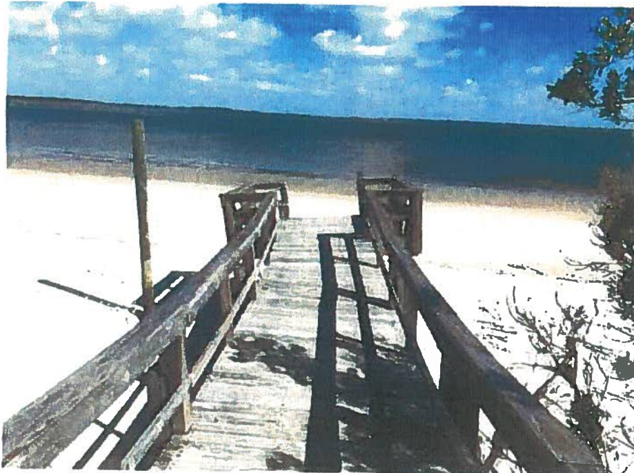
Figure 4 - Looking north towards beach. Obvious structural damage to 5.5' walk with 6" outside handrails.
