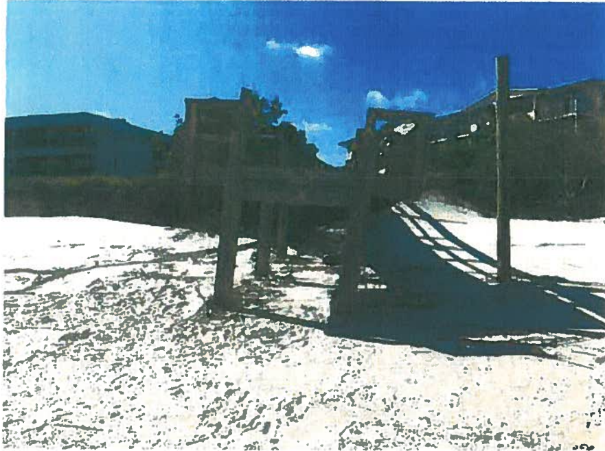
Figure 7 - Beach view of damaged walkway and 11.5' x 9.5' fixed deck. Stairs removed by storm.
