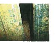
PHOTOGRAPH 2.6 OPEN JOINT IN PIPE 1
