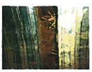
PHOTOGRAPH 2.8 OPEN JOINT IN THE CROWN OF PIPE 6
