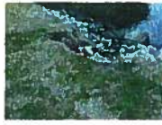
PHOTOGRAPH 1.7 EROSION AND FILTER FABRIC ADJACENT TO OUTFALL
