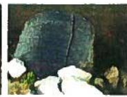
PHOTOGRAPH 1.2 FRACTURE AT THE UPSTREAM END OF PIPE 2
