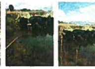
PHOTOGRAPH 1.9 TYPICAL UNDERSIZING OF THE PIPE AND FILTER FABRIC
