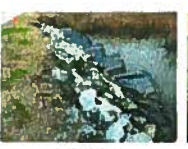
PHOTOGRAPH 2.5 DOWNSTREAM EMBANKMENT EROSION
