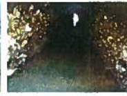
PHOTOGRAPH 1.8 SETTLEMENT OF THE RESPACED CONCRETE PIPE
