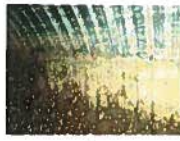
PHOTOGRAPH 1.4 4 FT LONG FRACTURE IN THE DOWNSTREAM END OF PIPE 4
