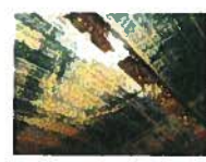
PHOTOGRAPH 2.7 OPEN JOINT IN PIPE 2
