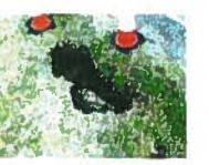
PHOTOGRAPH 2.3 SINKHOLE AT THE UPSTREAM END ABOVE PIPES 3 AND 5
