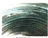
PHOTOGRAPH 2.4 CUT IN THE CROWN OF THE PIPE DUE TO FIBER OPTIC INSTALLATION - TYPICAL OF PIPES 1 THROUGH 7
