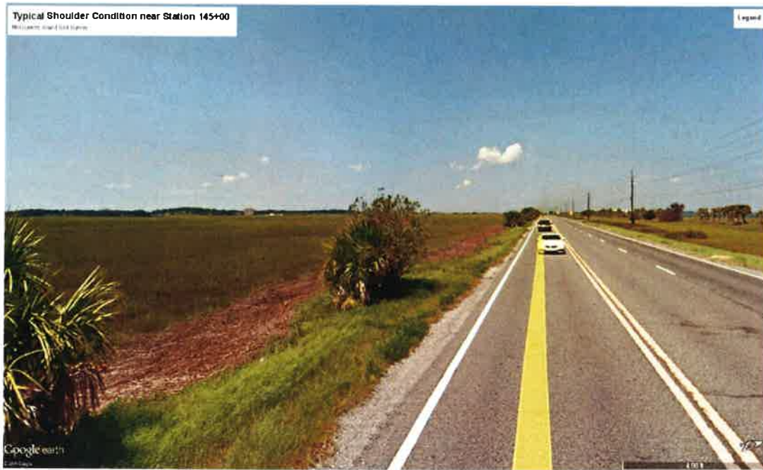
Photograph 4: Typical shoulder condition near Station 145+00 (see Drawing 11).
