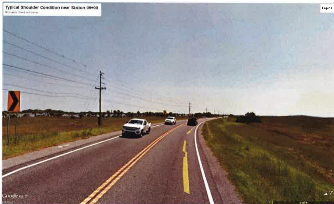
Photograph 3: Typical shoulder condition near Station 90+00 (see Drawing 7.)
