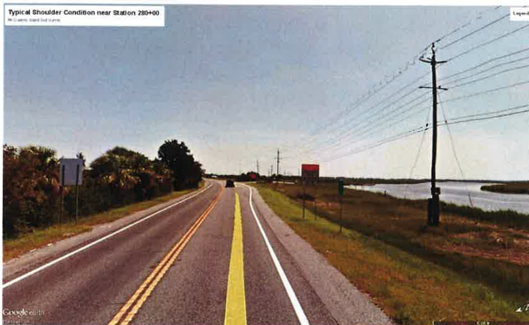
Photograph 5: Typical shoulder condition near Station 290+00 (see Drawing 22).
