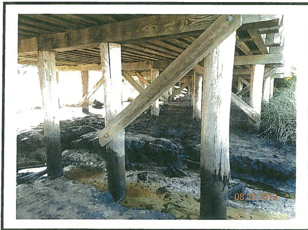
Photo 6: Tidally influenced damage to support piles.
