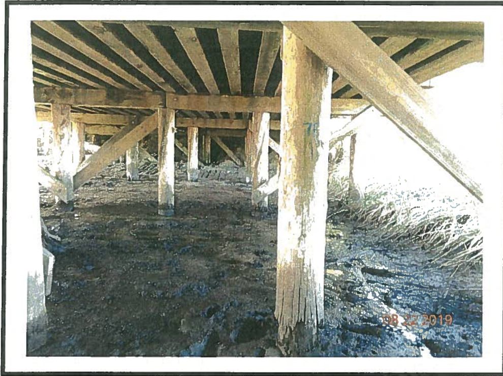
Photo 7: Tidally influenced damage to support piles
