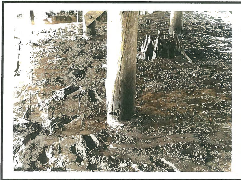
Photo 8: Tidally influenced damage to support piles.
