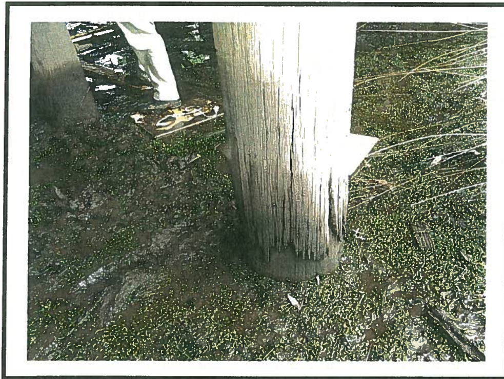
Photo 3: Tidally influenced damage to support piles
