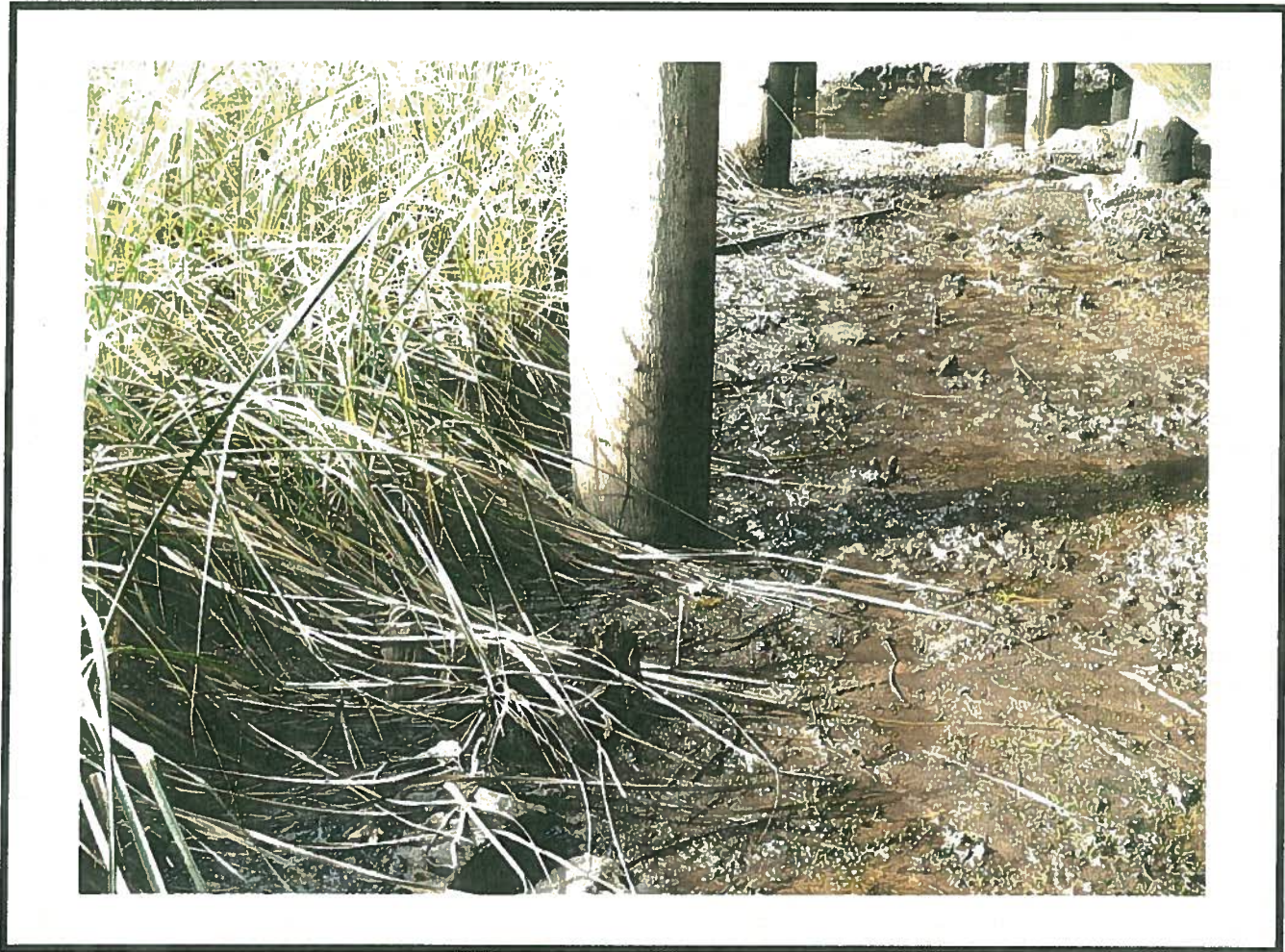
Photo 9: Tidally influenced damage to support piles
