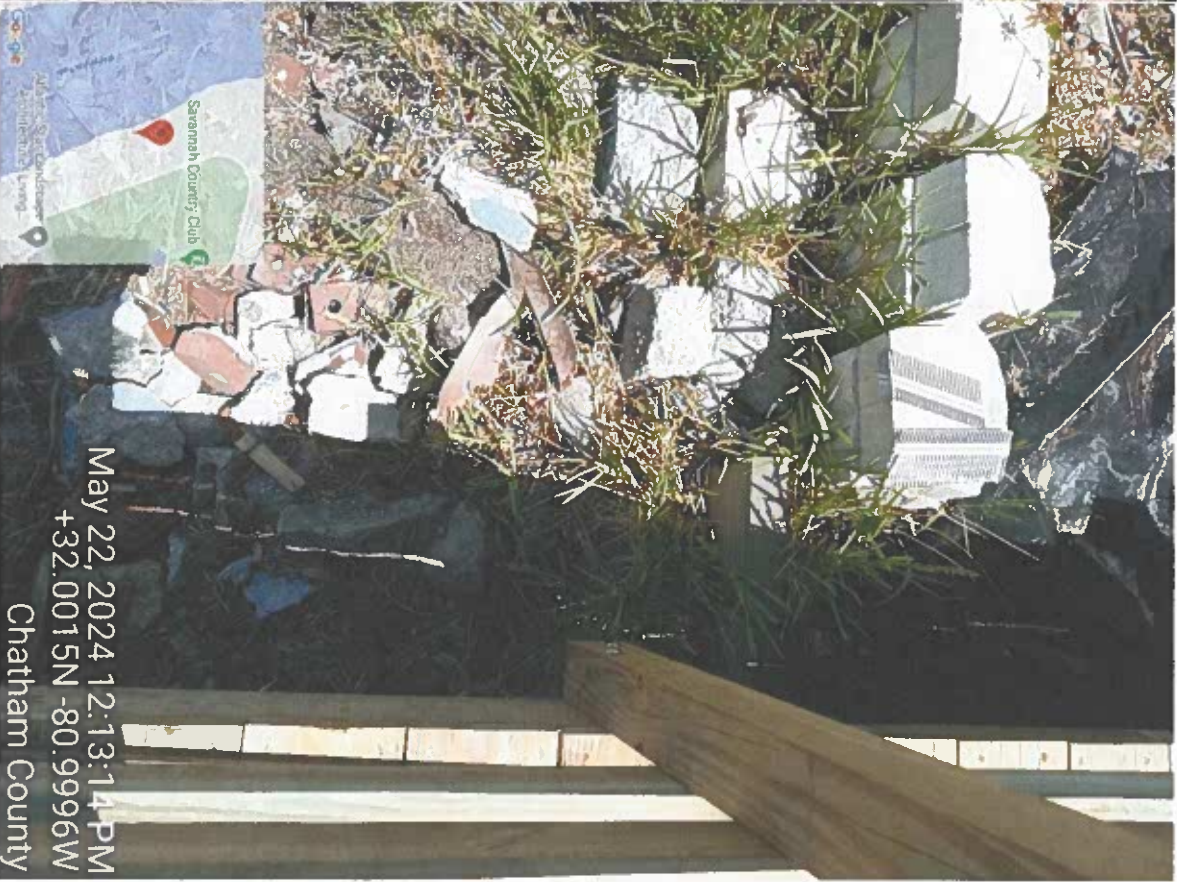
LOP20240039 – 736 Wilmington Island Road – Helgesen – Request for riprap maintenance
