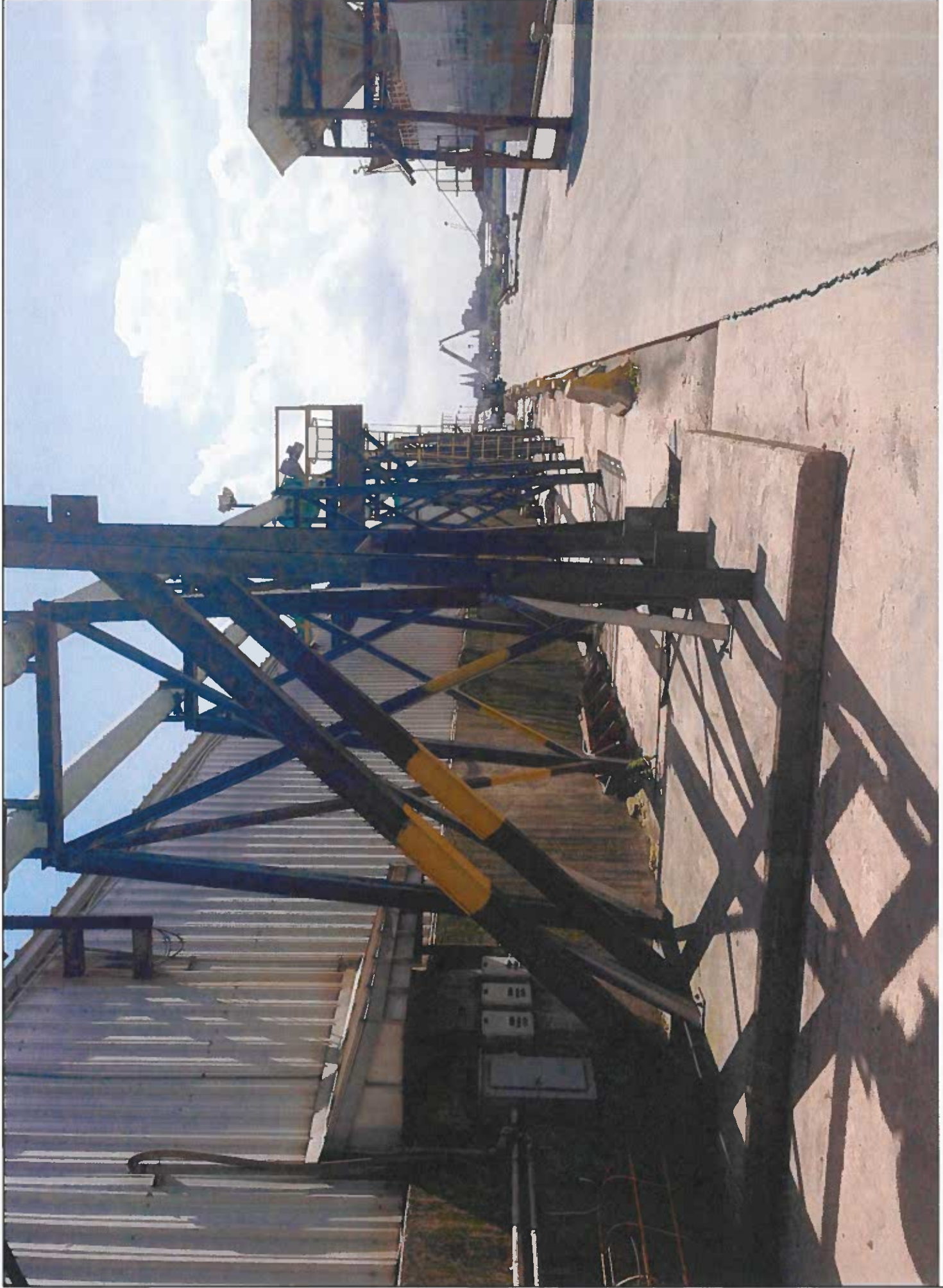
Photograph 3: This photograph was taken facing west and depicts the warehouse underwhich the bulkhead will be installed.
