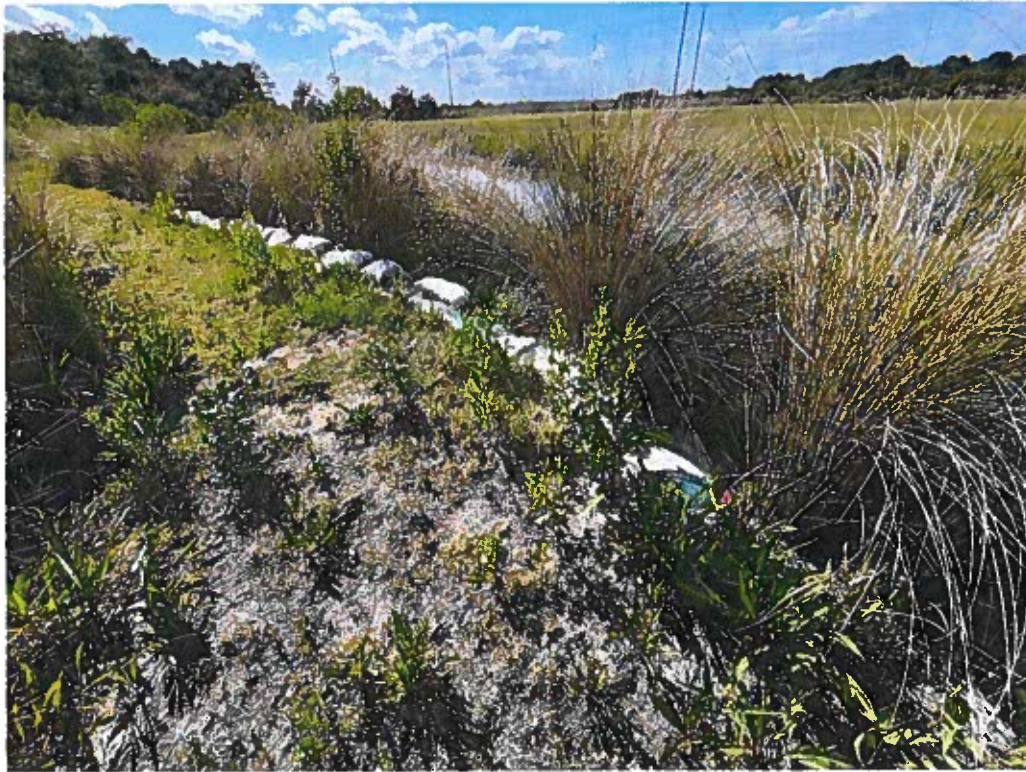
Photo 1: Area of documented increased erosion along dike, see temporary control structure installation
