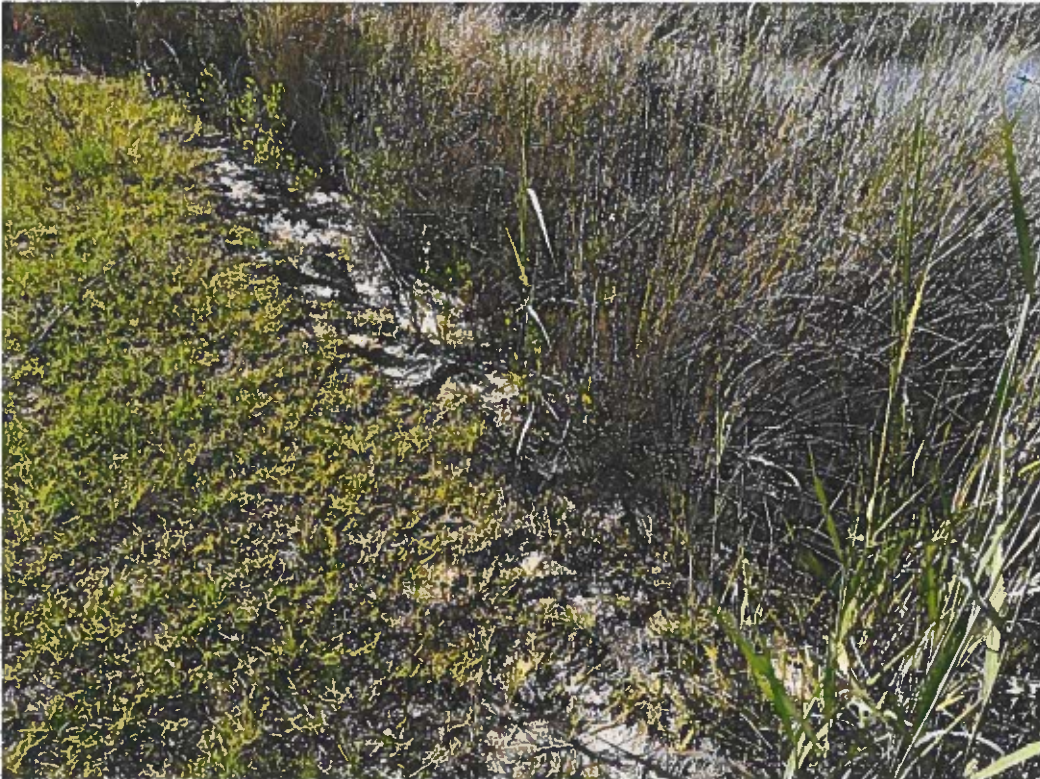
Photo 4: Area of additional erosion documented during dike inspections
