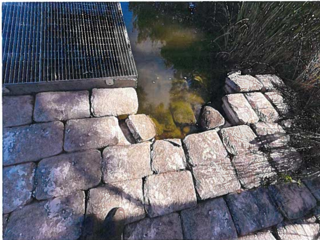
Photo 6: Failed cement bag rip rap located on west side of weir at control structure
