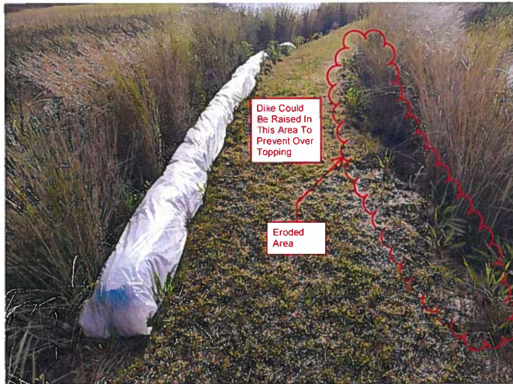
Erosion Tube That Has Been Placed on Dike Where Water Has Overtopped Dike
