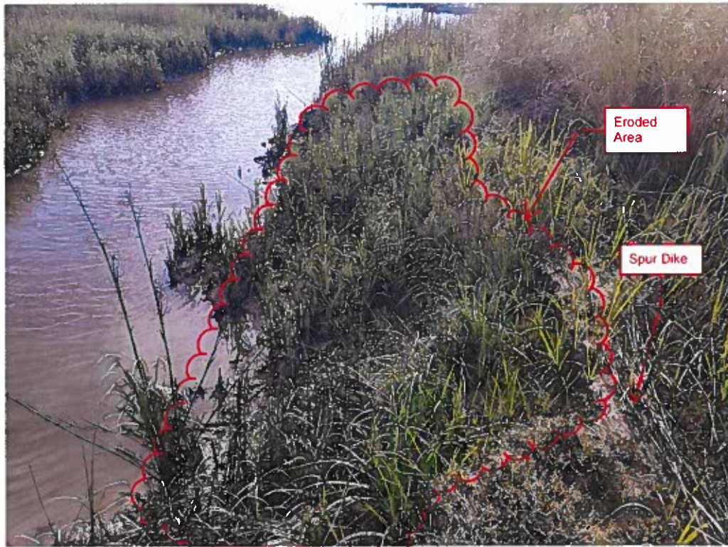
Erosion Along the Dike on The Marsh Side
