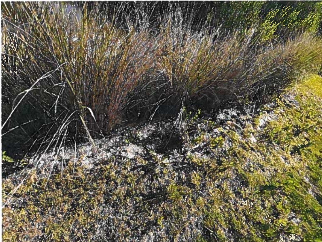
Photo 2: Area of ongoing erosion on southern side of dike, along the lagoon edge
