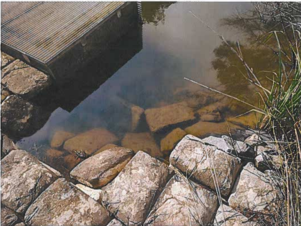
Slope Failure at The Lagoon Outlet Structure
