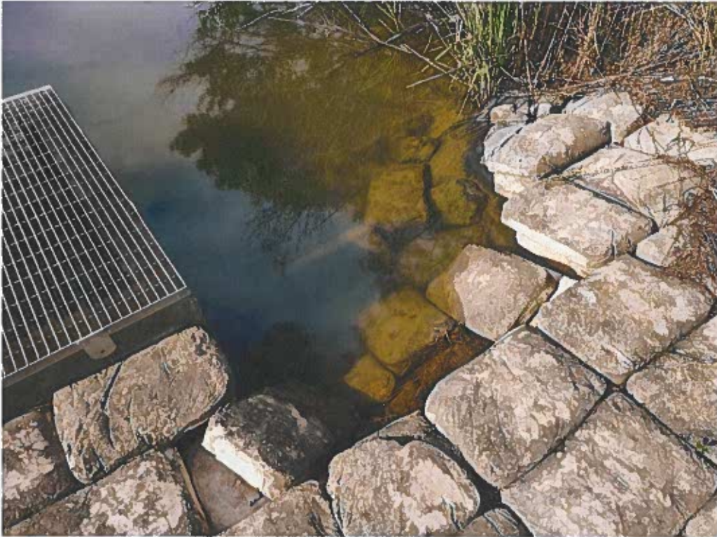
Slope Failure at The Lagoon Outlet Structure
