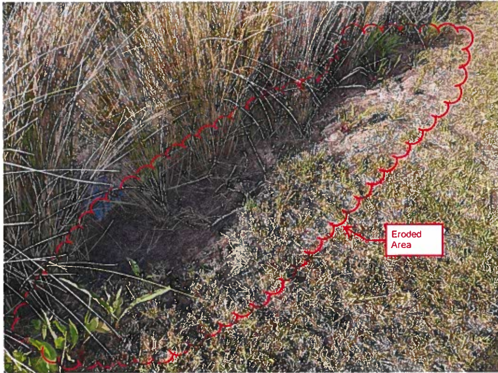
Erosion On the Lagoon Side of The Dike
