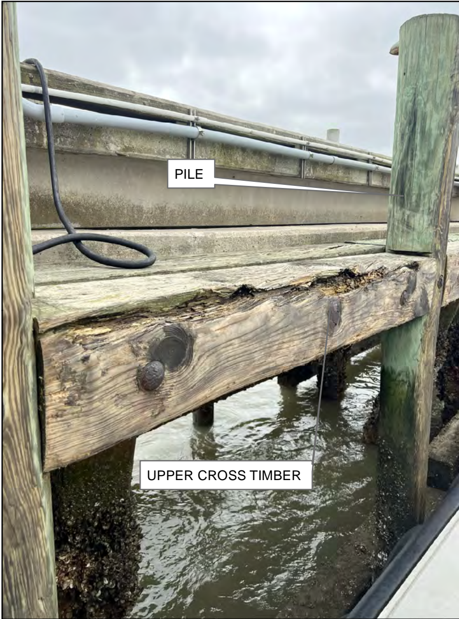
Photo 5: Example of upper cross timber and pile to be replaced
