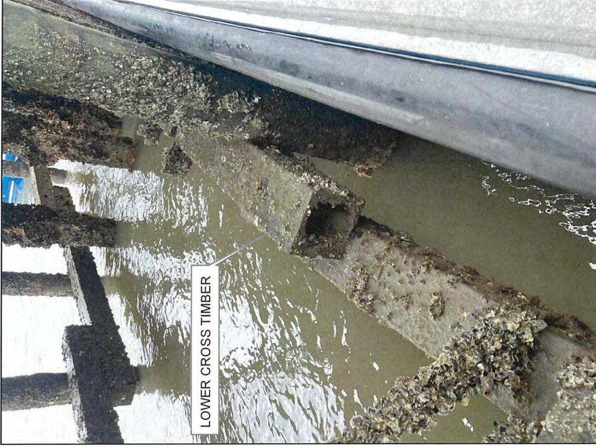
Photo 4: Example of lower cross timber to be replaced
