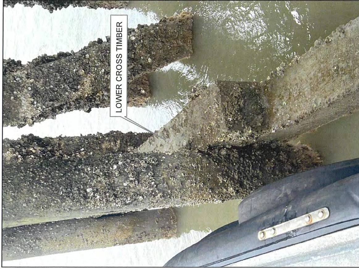
Photo 6: Example of lower cross timber to be replaced
