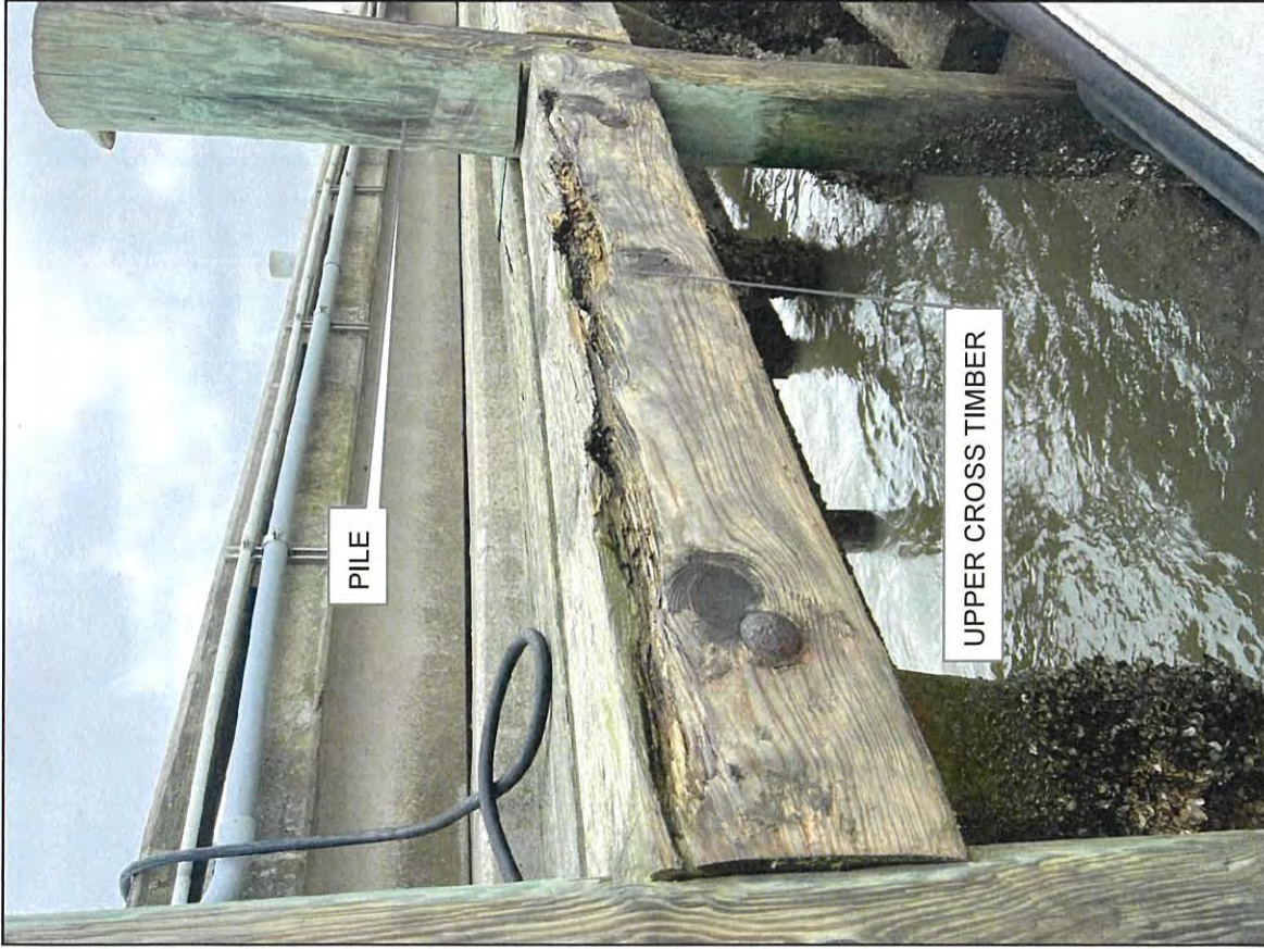
Photo 5: Example of upper cross timber and pile to be replaced
