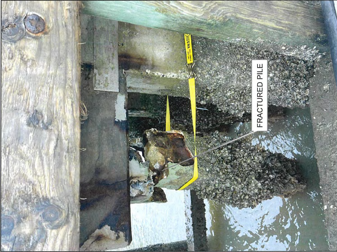
Photo 1 : Fractured concrete pile
