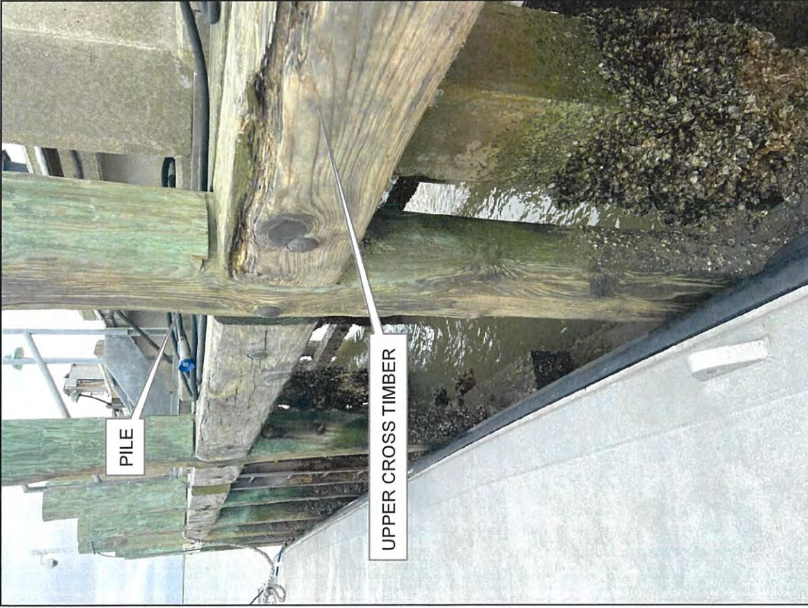
Photo 3: Example of upper cross timber and pile to be replaced
