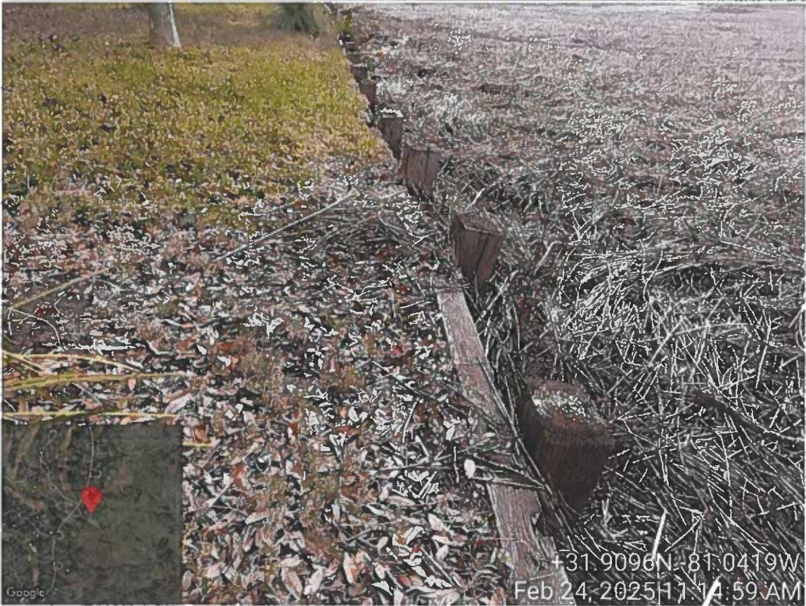
Site visit – 2 Laurel Hill Lane – Yeager – LOP Request bulkhead replacement – PM Cheyenne Osborne w/ Mariana S.
