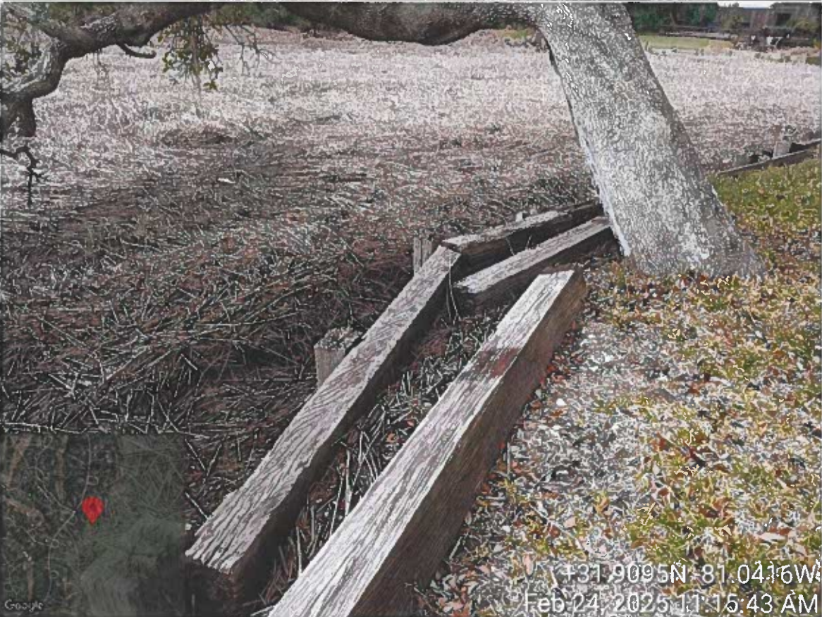
Site visit – 2 Laurel Hill Lane – Yeager – LOP Request bulkhead replacement – PM Cheyenne Osborne w/ Mariana S.
