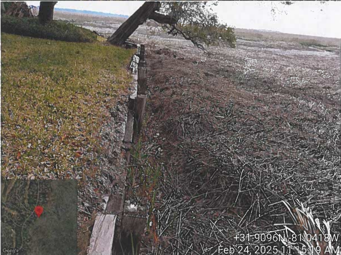
Site visit – 2 Laurel Hill Lane – Yeager – LOP Request bulkhead replacement – PM Cheyenne Osborne w/ Mariana S.
