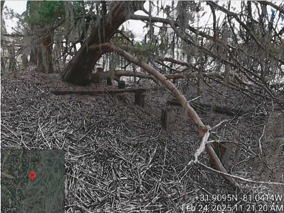
Site Visit – 3 Laurel Hill Road – Collins – LOP Request replace bulkhead – PM Cheyenne Osborne w/ Mariana S.
