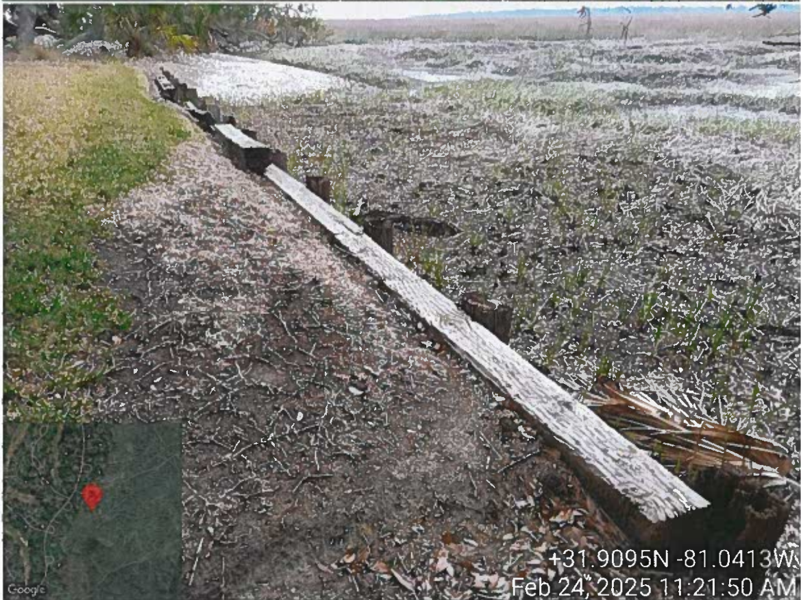
Site Visit – 3 Laurel Hill Road – Collins – LOP Request replace bulkhead – PM Cheyenne Osborne w/ Mariana S.
