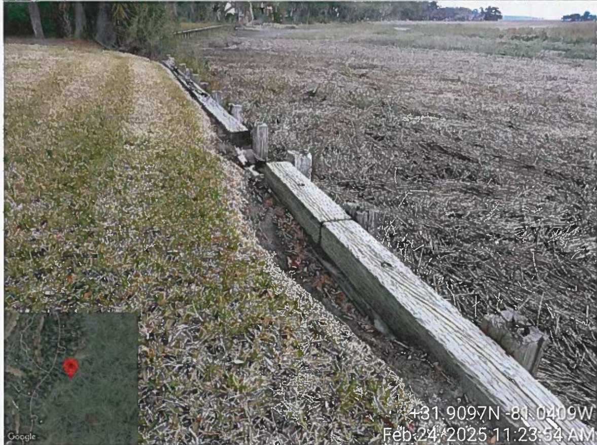
Site Visit – 3 Laurel Hill Road – Collins – LOP Request replace bulkhead – PM Cheyenne Osborne w/ Mariana S.
