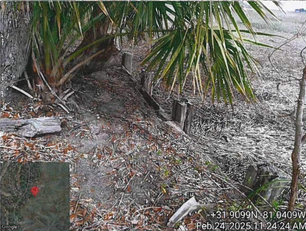
Site Visit – 3 Laurel Hill Road – Collins – LOP Request replace bulkhead – PM Cheyenne Osborne w/ Mariana S.
