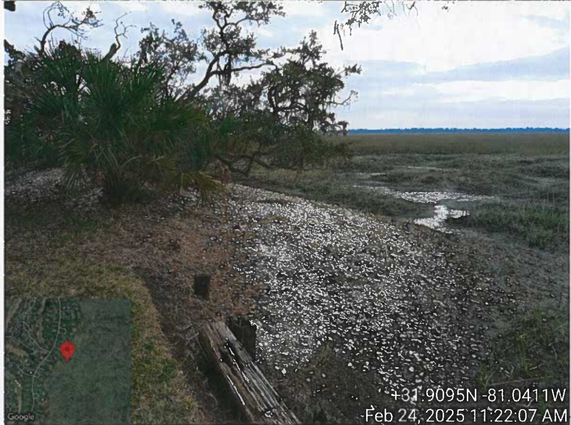
Site Visit – 3 Laurel Hill Road – Collins – LOP Request replace bulkhead – PM Cheyenne Osborne w/ Mariana S.
