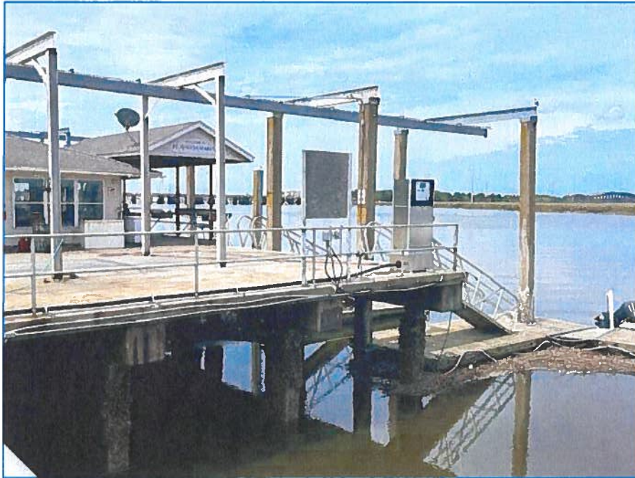
Existing piles and docks to be replaced
