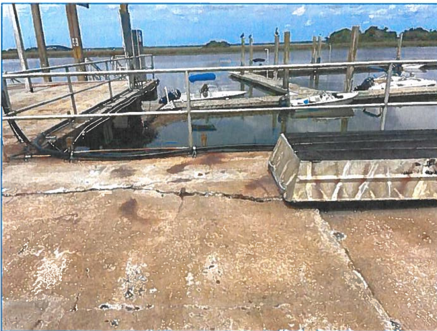
Facing west at existing bulkhead showing concrete cracking
