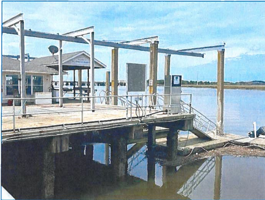
Existing piles and docks to be replaced
