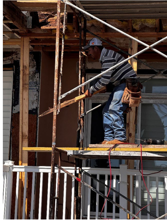
Photo of Rot around Door
