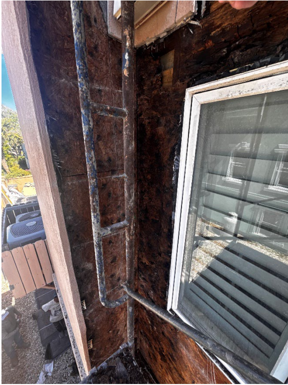
Photo of Rot around Windows
