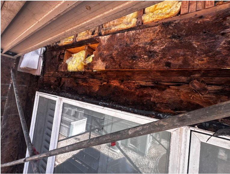
Photo of Rot around Windows
