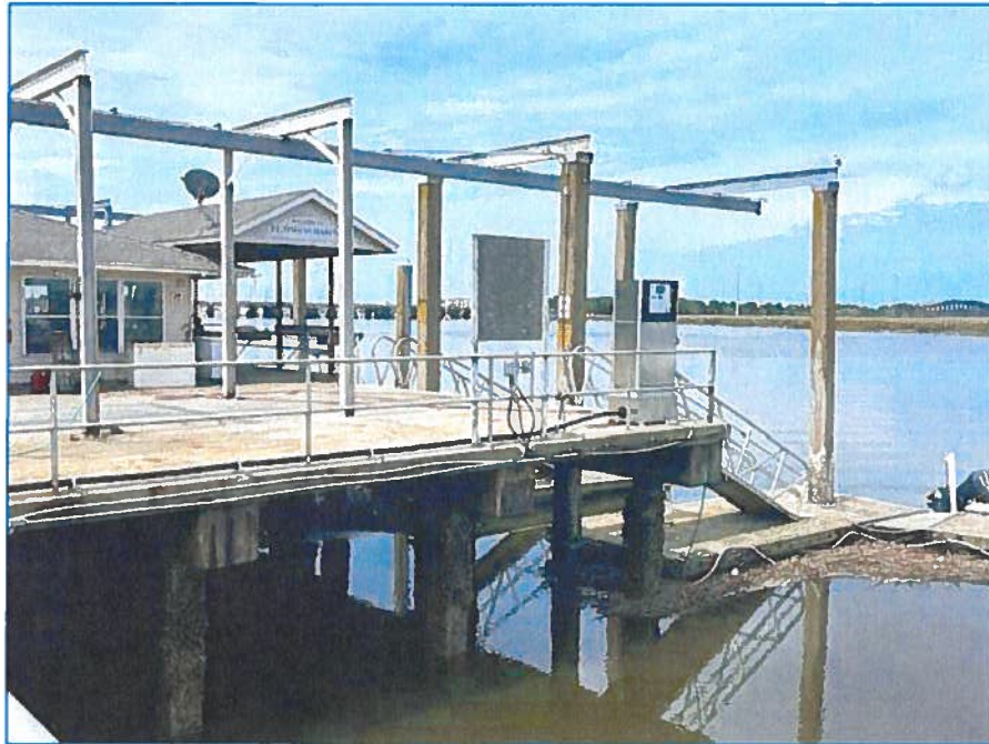
Existing piles and docks to be replaced
