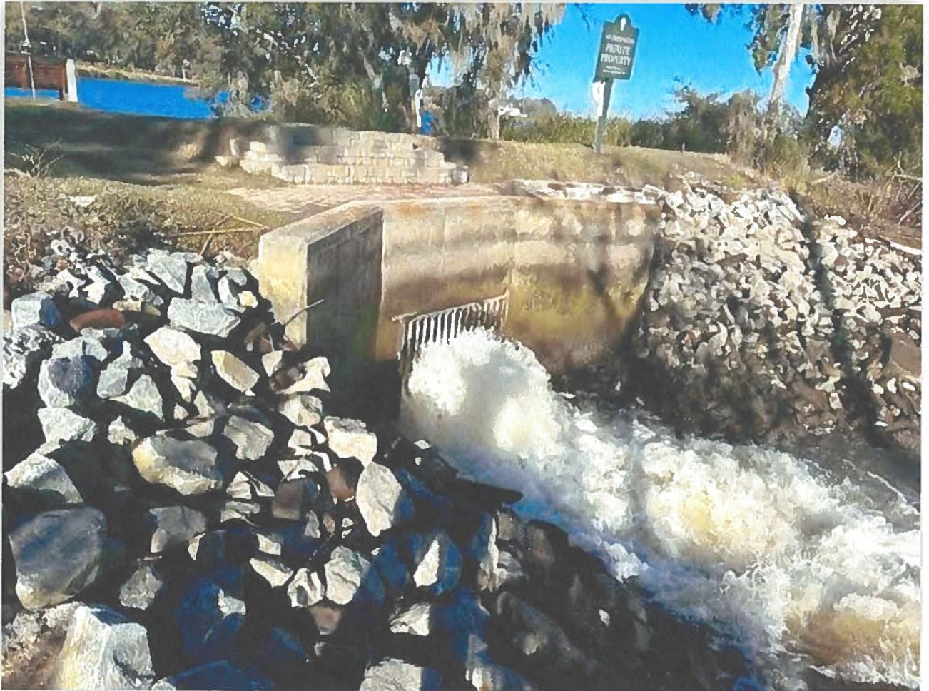
Figure 28. Control Structure #3-This structure has by far the largest outfall of all three structures.
