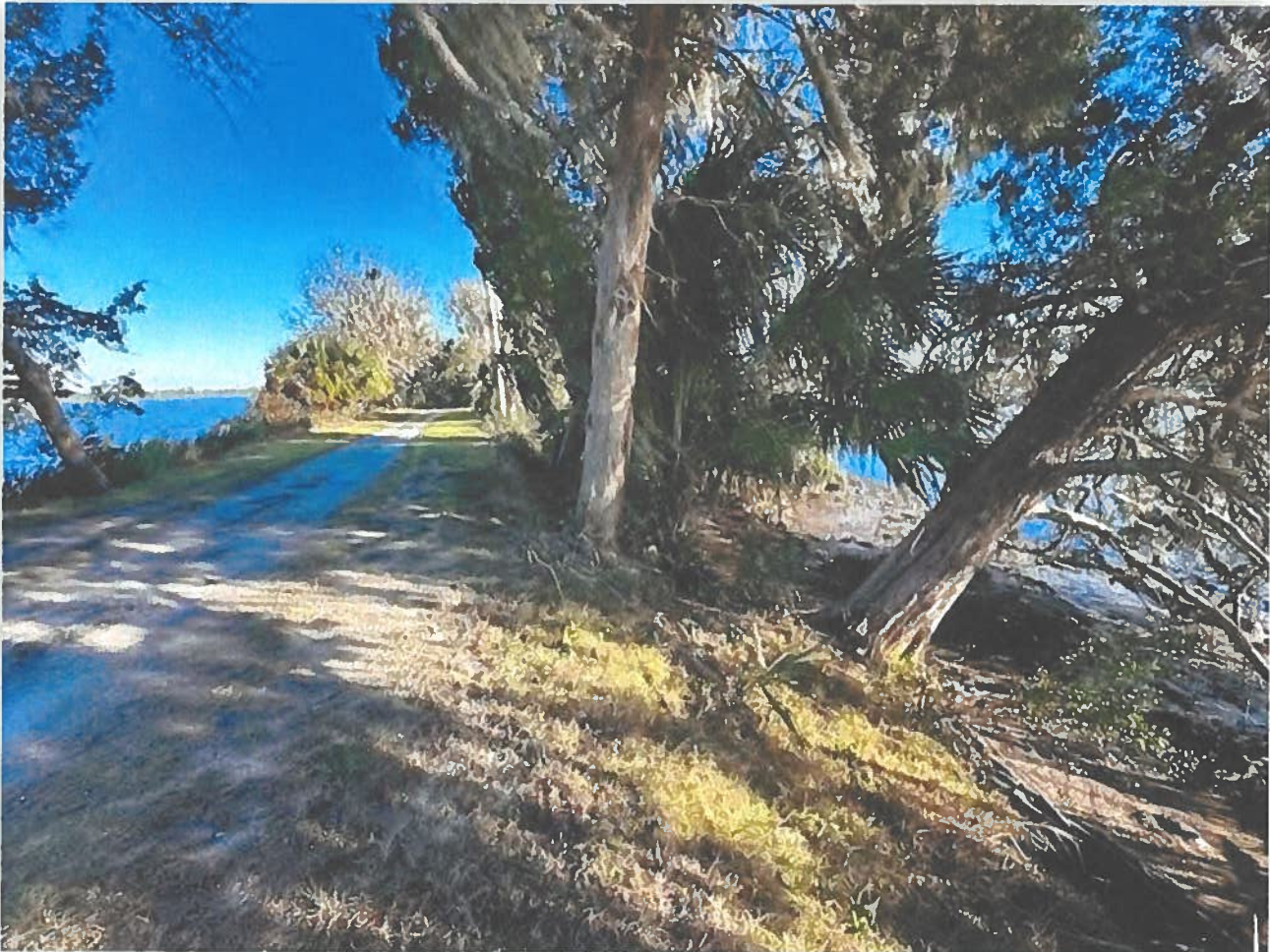
Figure 24. Narrow Section of Levee recommended for riprapping.
