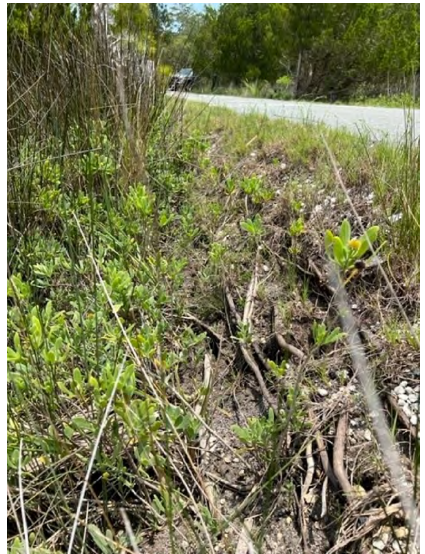
Photo 2: Road shoulder erosion
