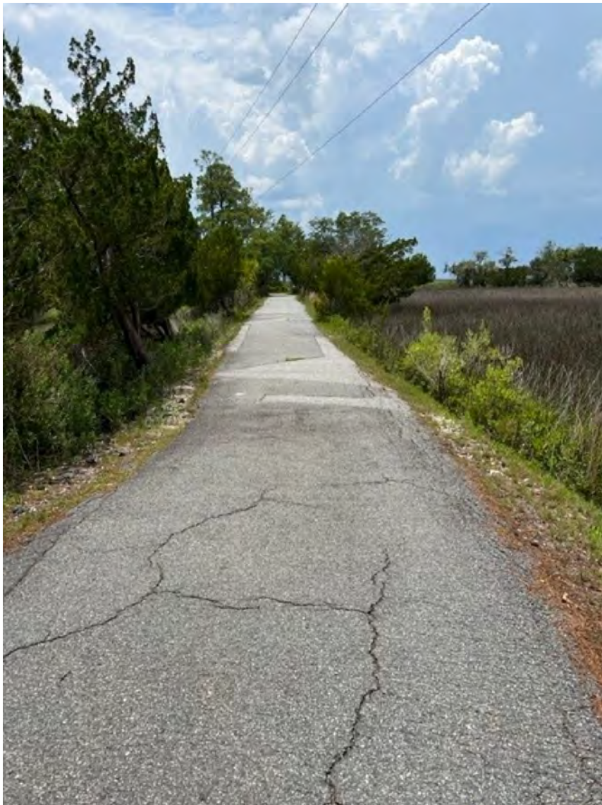
Photo 1: Existing causeway facing west. Note cracking road surface
