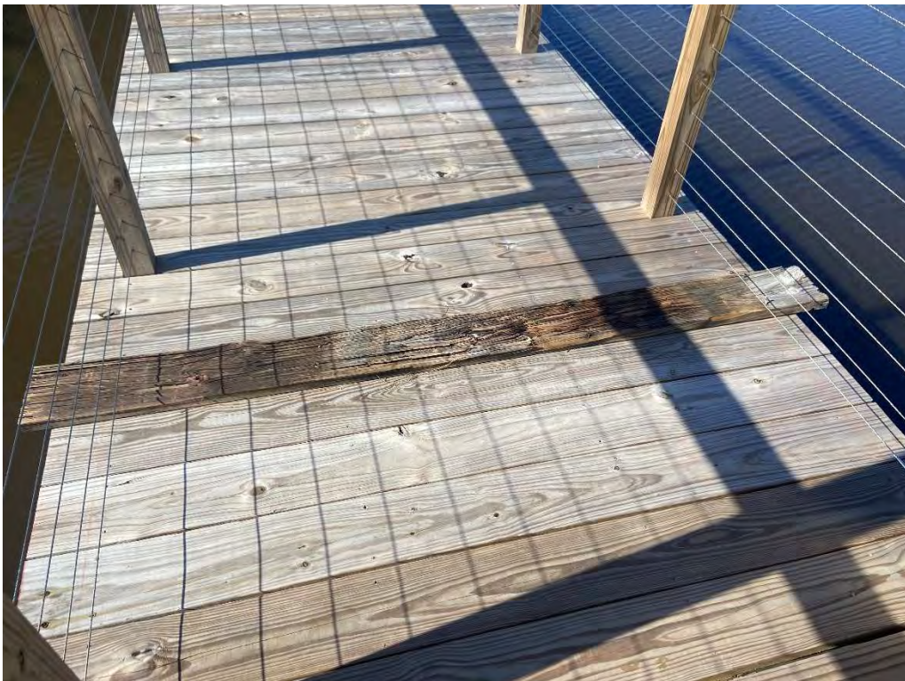
Photo 8: Example of original boards vs replacement 7' boards
