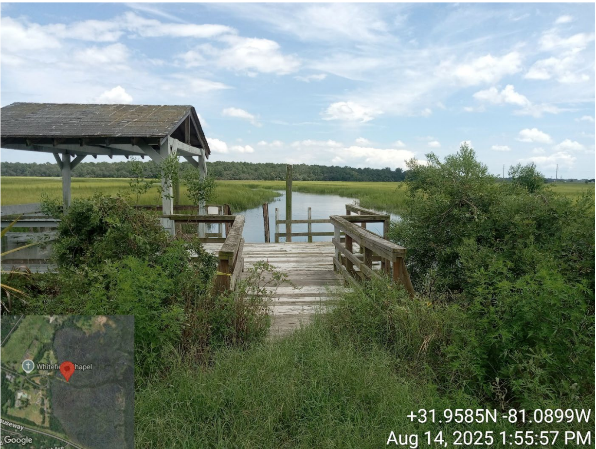
Site Visit – CMP20250040 – 9520 Ferguson Ave – replace dock – PM Cheyenne Osborne w/ Chelsea K.
