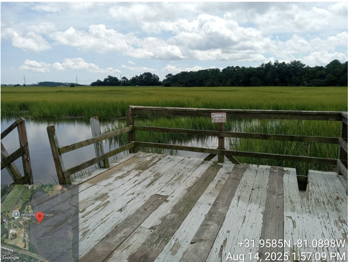
Site Visit – CMP20250040 – 9520 Ferguson Ave – replace dock – PM Cheyenne Osborne w/ Chelsea K.
