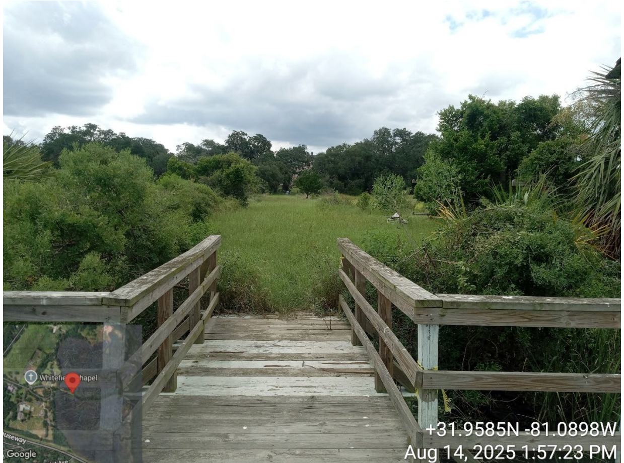
Site Visit – CMP20250040 – 9520 Ferguson Ave – replace dock – PM Cheyenne Osborne w/ Chelsea K.
