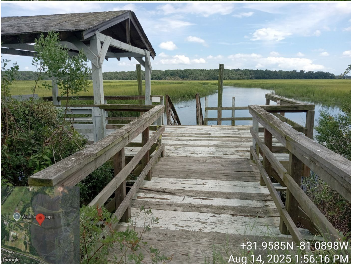
Site Visit – CMP20250040 – 9520 Ferguson Ave – replace dock – PM Cheyenne Osborne w/ Chelsea K.
