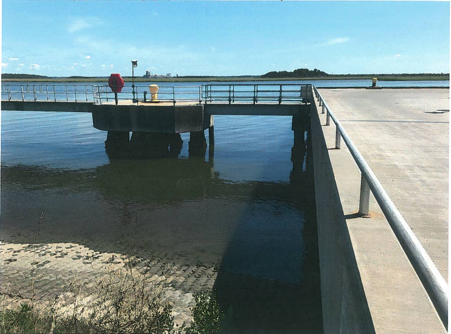
Photograph 1: Location of proposed 63' x 164' deck extension on the upstream end of Berth 2
