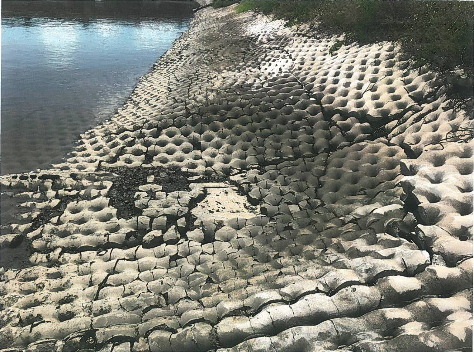
Photograph 3: Example of damaged concrete revetment to be repaired
