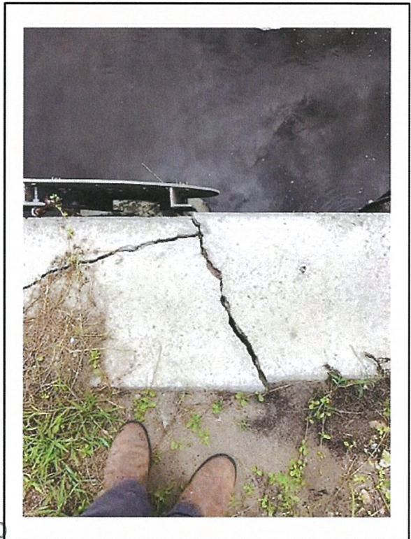
West Culvert: Concrete Wall Damages
