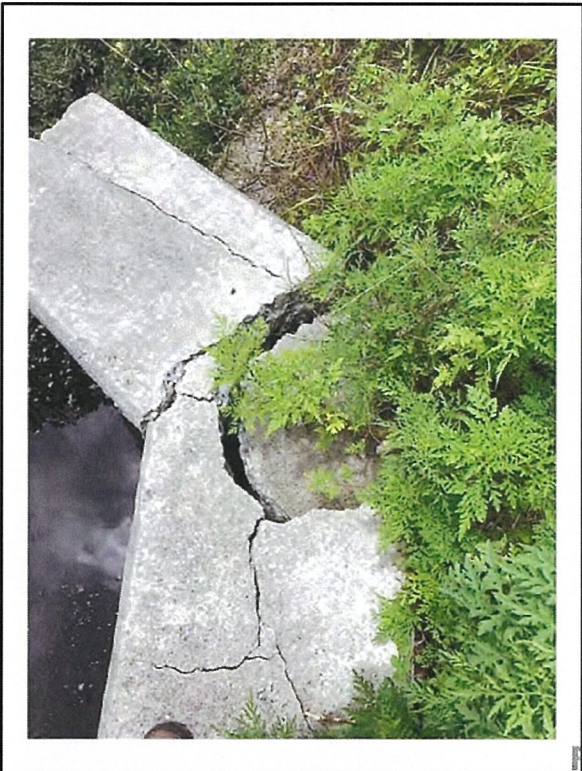
West Culvert: Concrete Wall Damages
