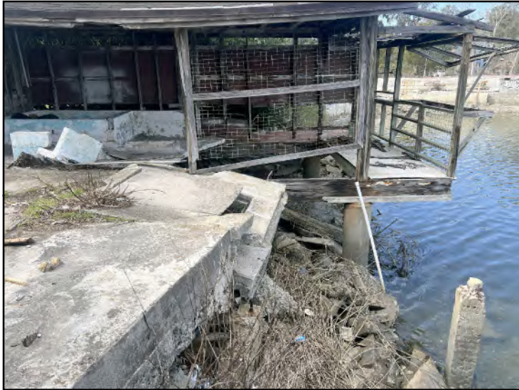
Photo 1: Existing wall and broken concrete
