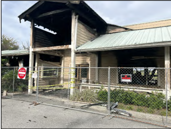
Photo 1: Existing restaurant condition after fire
