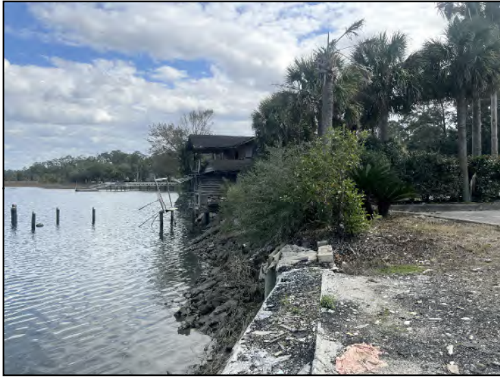
Photo 1: Existing wall and broken concrete
