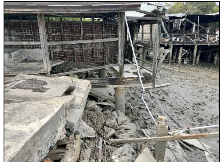
Photo 8: Old bait well to be removed at 7012 LaRoche
