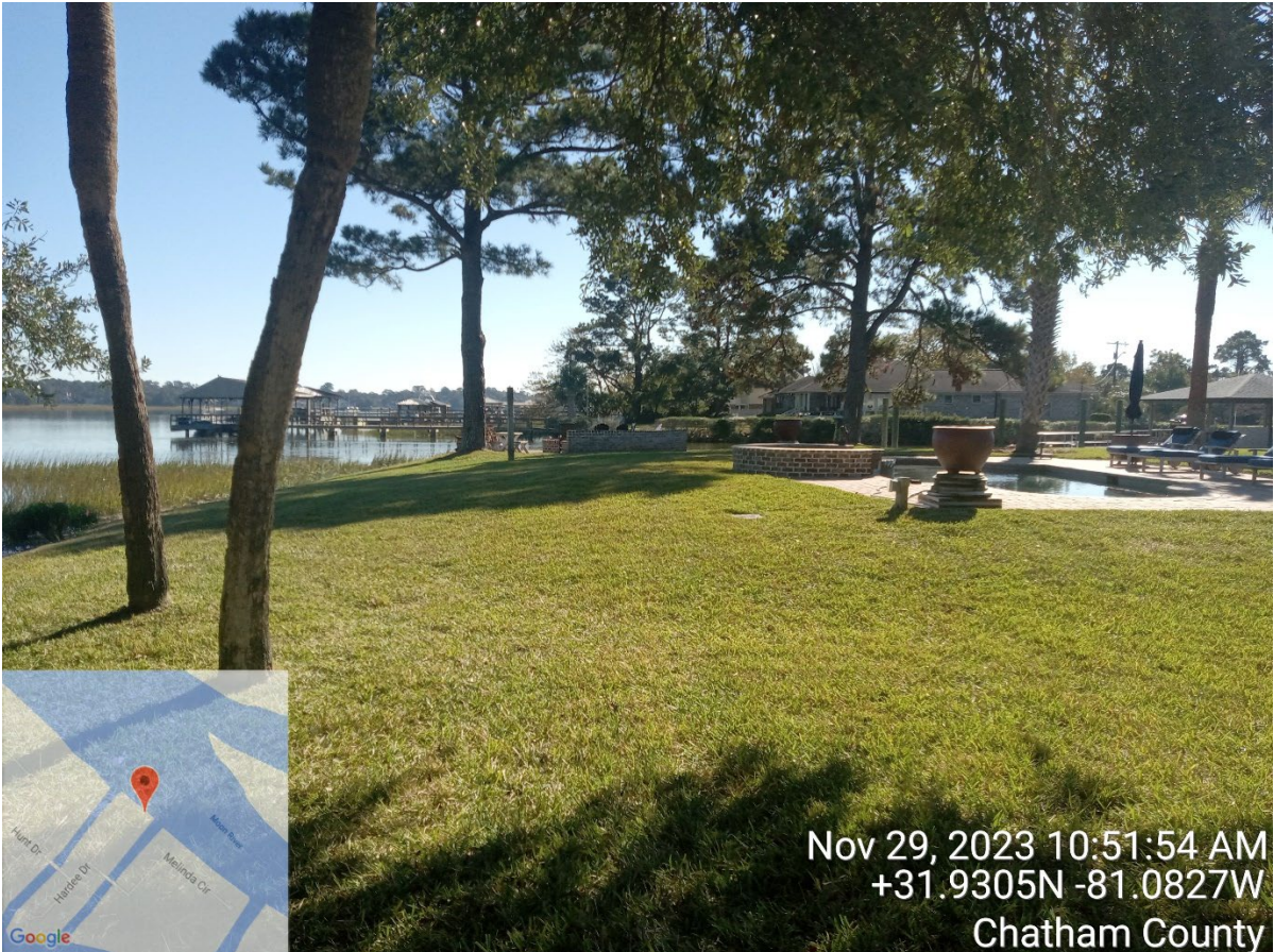
Site Visit – 11.29.23 – 13 Hardee Drive – Chuck Hartman – CMPA Bulkhead along Moon River By Cheyenne Osborne w/ Maitland Bass
