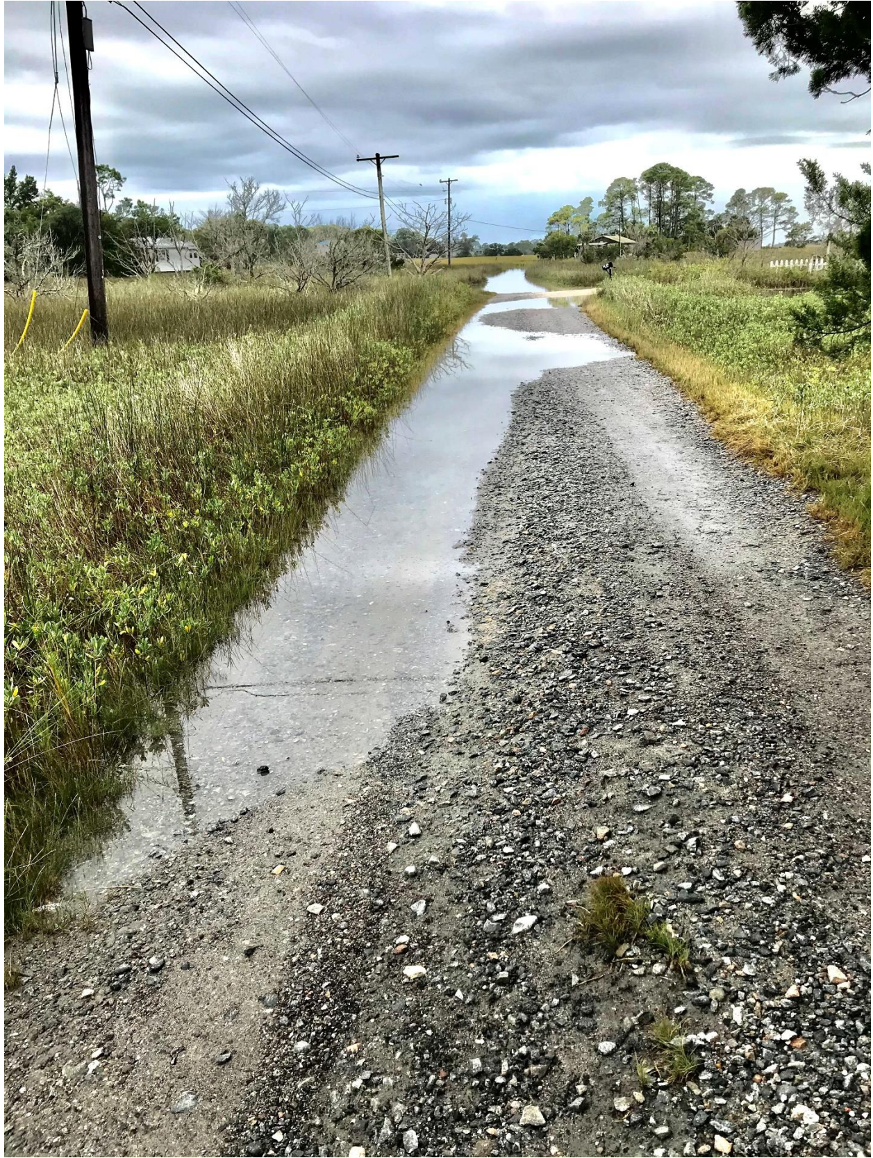
October 21, 2020 around High Tide: Looking north from Polk Street ROW toward US 80
