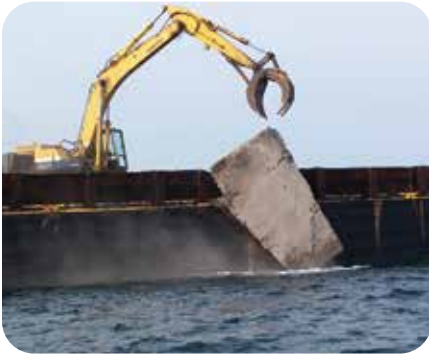
Concrete rubble very closely mimics the natural hard bottom found in GA.
